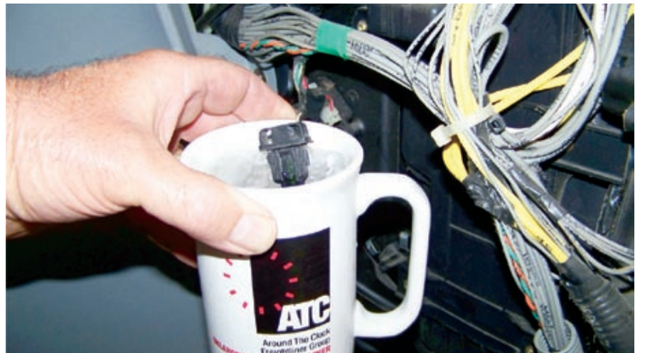
Figure 2 - Testing the Evap Temp Sensor in an Ice Bath
